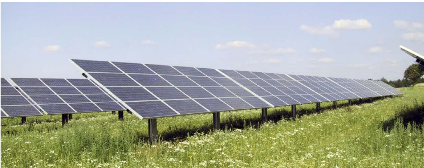
Fig. 7: Typical ground-mounted PV system. © Fraunhofer ISE
