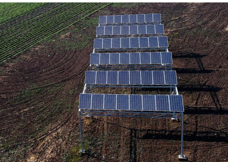
Fig. 19: Pilot PV systems in Curacaví and Lampa where the Fraunhofer Chile Research Institute is investigating which crops benefit from slightly less solar radiation. © Fraunhofer Chile
